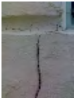
Cracked due to existing paint underneath
